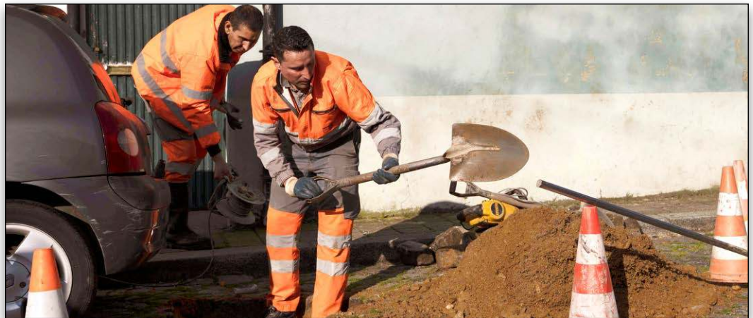
Maintenance quickly respond to issues and update system information while in the field.
